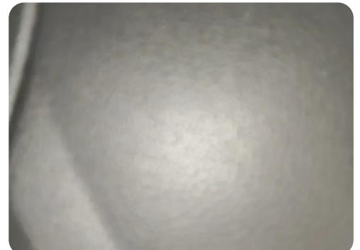
RF Door Trim: Scratches present
