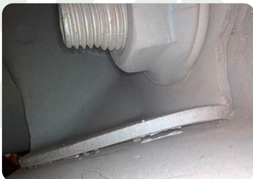
RF Long. Member Flange: Deformation \geq 3\text{ cm}^2 present
